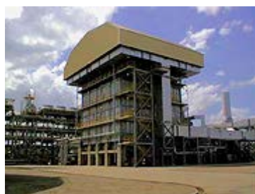
Trinidad steam reformer.
